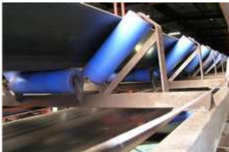
Gambar 4 Carry Roller terpasang di frame conveyor
